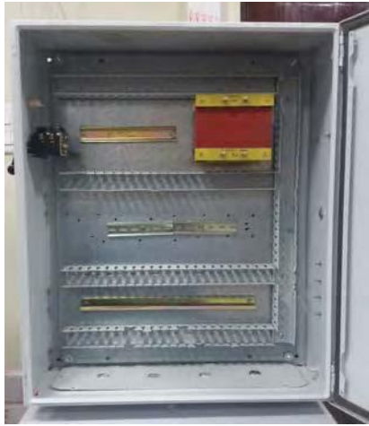
CONTROL PANEL WITH RACEWAYS/DIN RAILS
